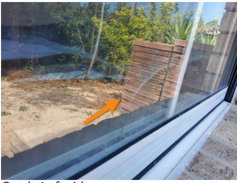
Crack. Left side
