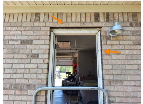
Garage door needs recalling. Growth present
