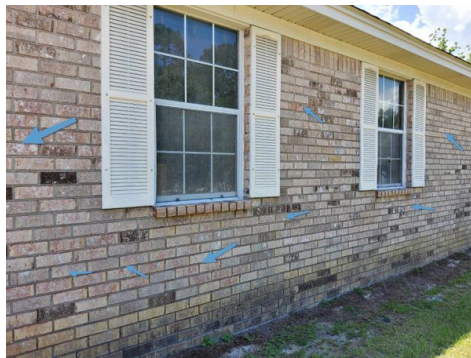
Multiple locations at garage
