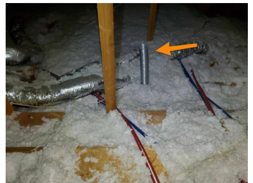
Venting moisture into attic
