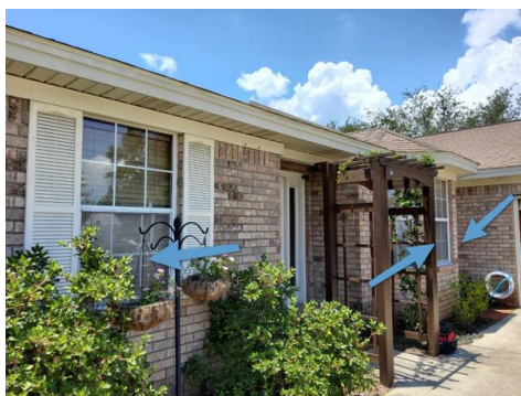
3 screens damaged at front
